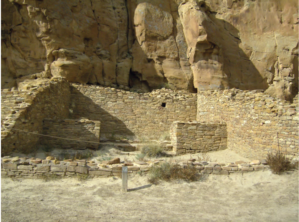
Figure 8. A 2010 photograph by Mathien that illustrates that the doorway in north wall of Room 8 has been filled in completely. The cliff-face stairway continues to erode and is barely discernible today.
